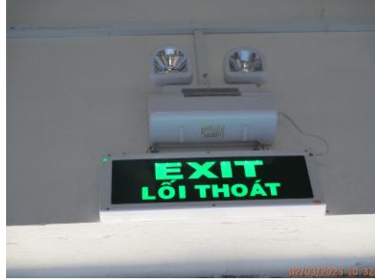
28. Exit sign and emergency light.jpg
