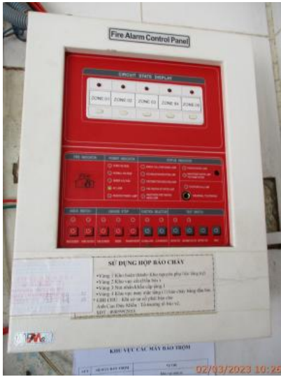
19. Fire alarm control panel.jpg
