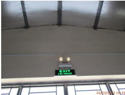
29. Emergency light testing onsite.jpg
