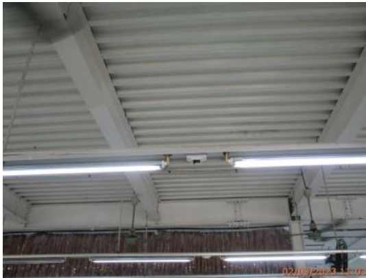
63. Electrical wire in good condition.jpg
