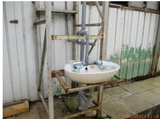
70. Eye wash equipment.jpg
