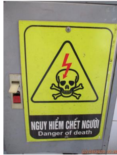
32. Dangerous warning sign.jpg
