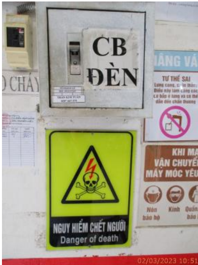
39. Electrical panel with dangerous warning sign posted.jpg
