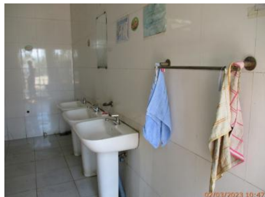
48. Hand washing area at toilet with soap.jpg
