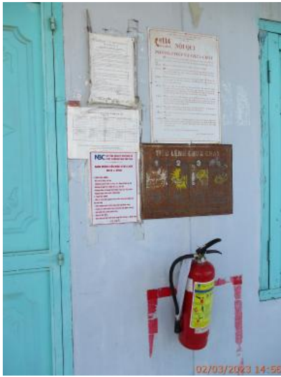
79. Dormitory for employee - fire extinguisher.jpg
