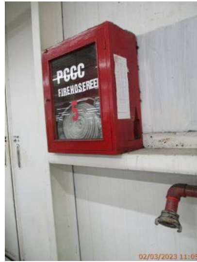
24. Fire hose reel and fire hydrant.jpg
