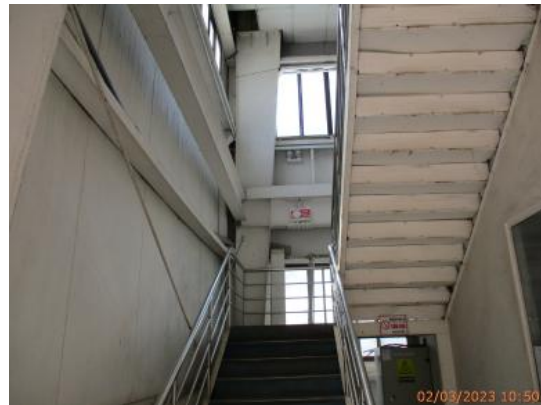
52. Emergency light equipped at the stairwell.jpg
