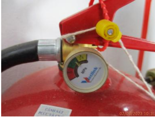
23. Fire extinguisher in good condition.jpg
