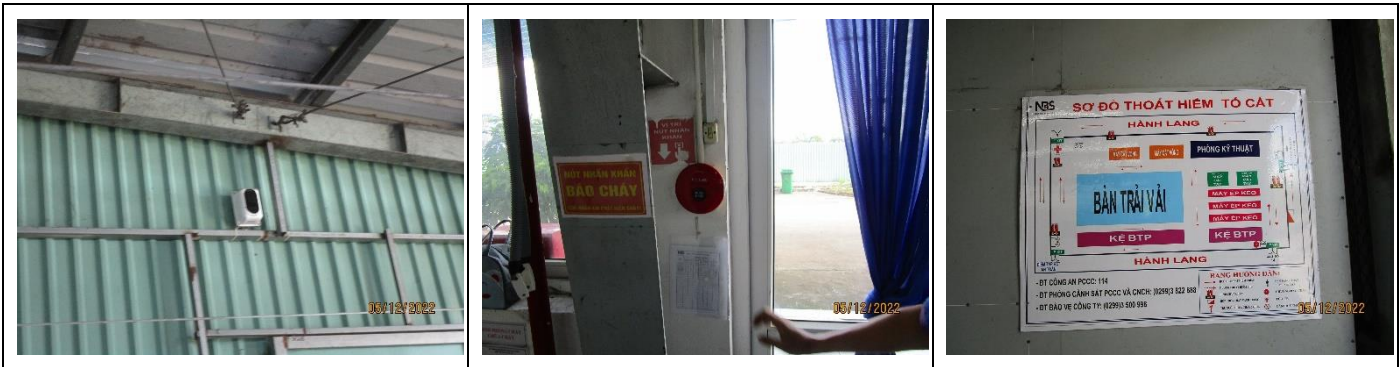
Automatic fire alarm central Assembly point Sprinkler system at production areas
